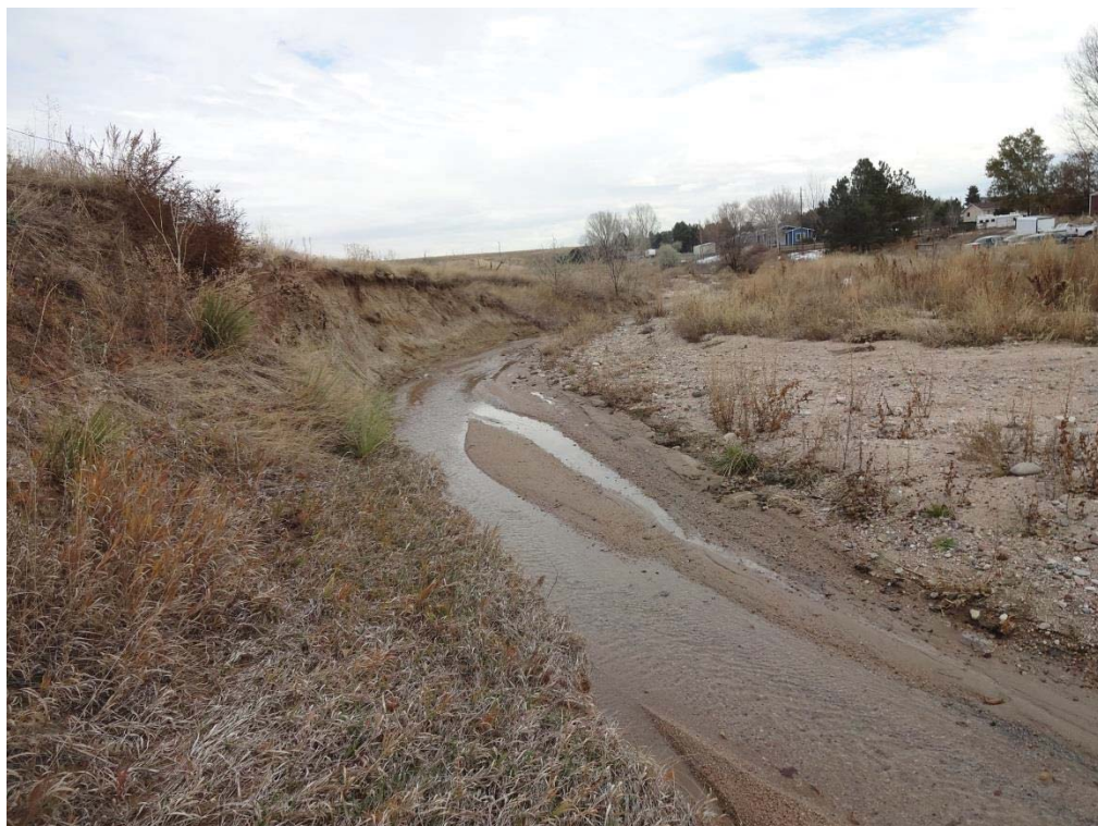
Photo4. View of the upstream segment of Happy Canyon Creek near the private residences. The cut bank and the sandy soils are precluding the establishment of wetland vegetation.
