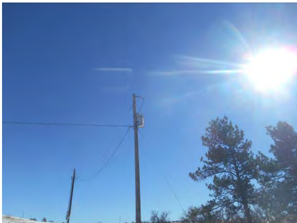
Photo #9 View of a pole-mounted transformer observed near the northwest corner of the site. View to the north.
