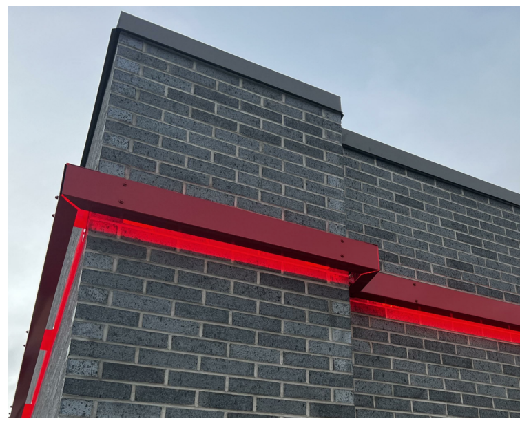
BACK-LIT BANDING; REF TR-1 FOR COLORS NOTE: PHOTO IS INTENDED TO DISPLAY THE RED BANDING AND LIGHT SOURCE AND NOT REPRESENT THE BUILDING MATERIALS FOR THIS PROJECT LOCATION AS CHANGES MAY OCCUR AS REQ'D PER THE LOCAL AHJ.
