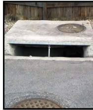
Denver No. 14 Curb Opening
