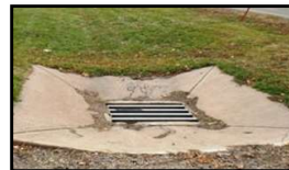
CDOT Type C Inlet In Depression
