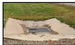
CDOT Type C Inlet In Depression
