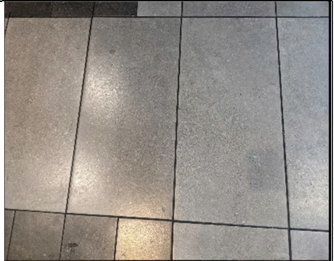
HA# 02 | Black Grout associated with Ceramic Floor Tile
