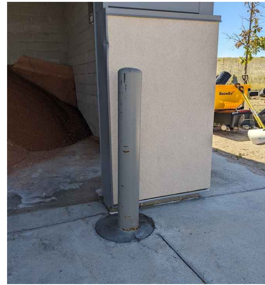
4 MATERIAL: CONCRETE FILLED SCHEDULE 40 STEEL COLOR: SP1 - LIGHT GRAY RE-ARCHITECTURAL PIPE BOLLARD EXAMPLE IMAGE - LOADING DOCK AND SHED 09 of 25 NO SCALE
