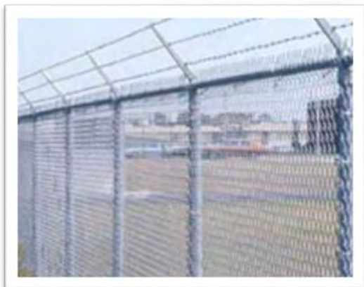
Un-coated Chain Link Prohibited
