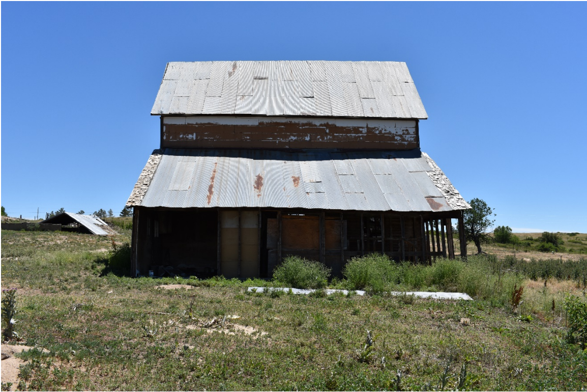
5DA875 – House (F1) west elevation; view to the east. Photograph: DSC_0214 Date: 6/25/2018
