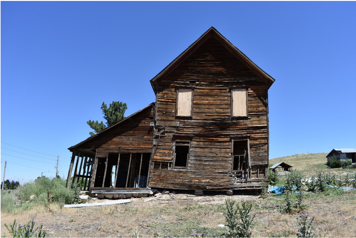
5DA875 – House (F1) south elevation; view to the north. Photograph: DSC_0223 Date: 6/25/2018
