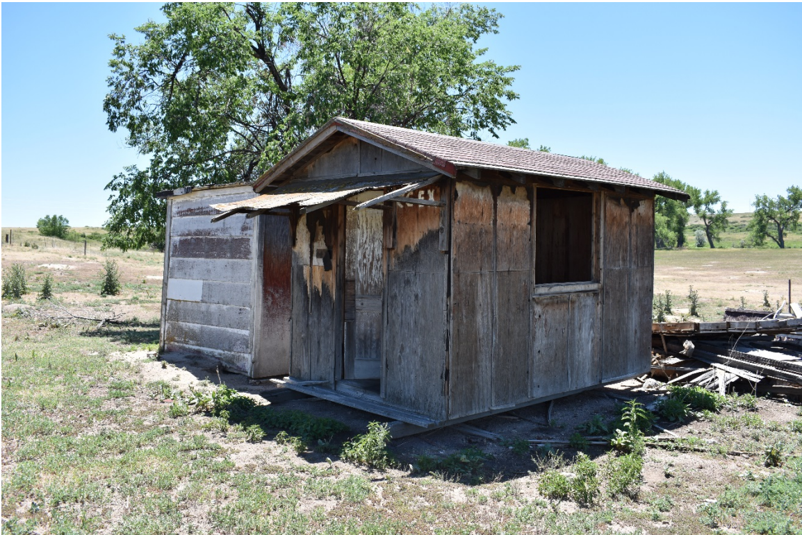
5DA875 – Overview of outbuildings F8 and F9; view to the southeast. Photograph: DSC_0261 Date: 6/25/2018
