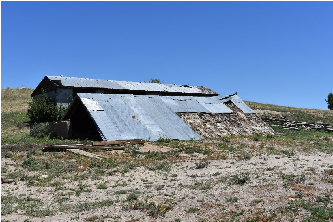
5DA875 – Collapsed barn (F5); view to the north-northeast. Photograph: DSC_0246 Date: 6/25/2018
