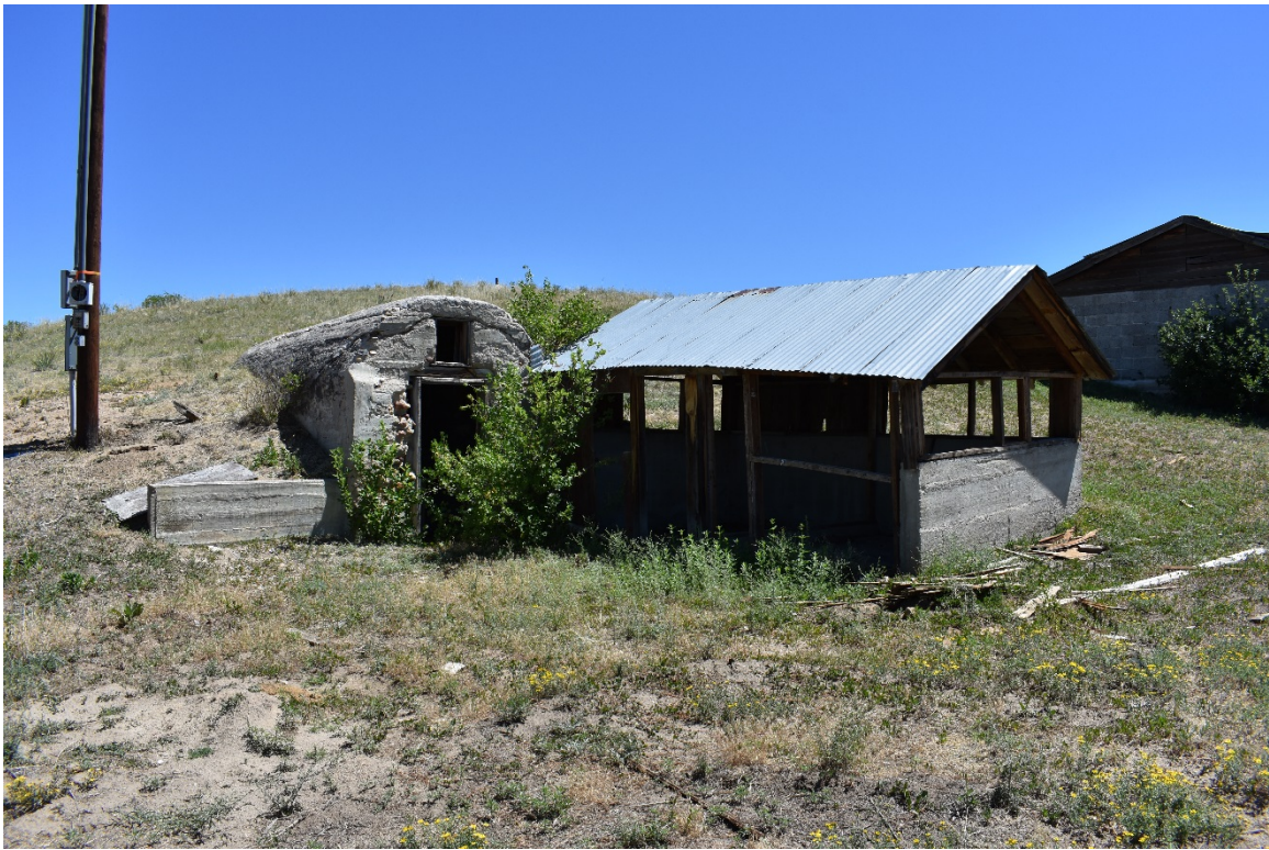
5DA875 – Overview of root cellar (F2) and outbuilding (F3); view to the northeast.
