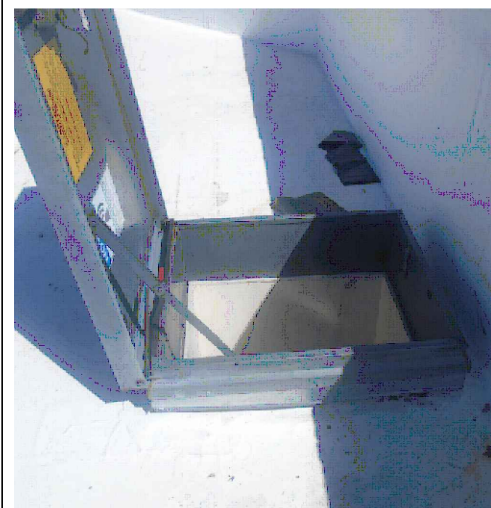
1 ROOFTOP ACCESS HATCH
